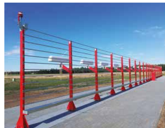
Fot: Systemy nowiny ILSLOC (Instrument Landing System localizer)
